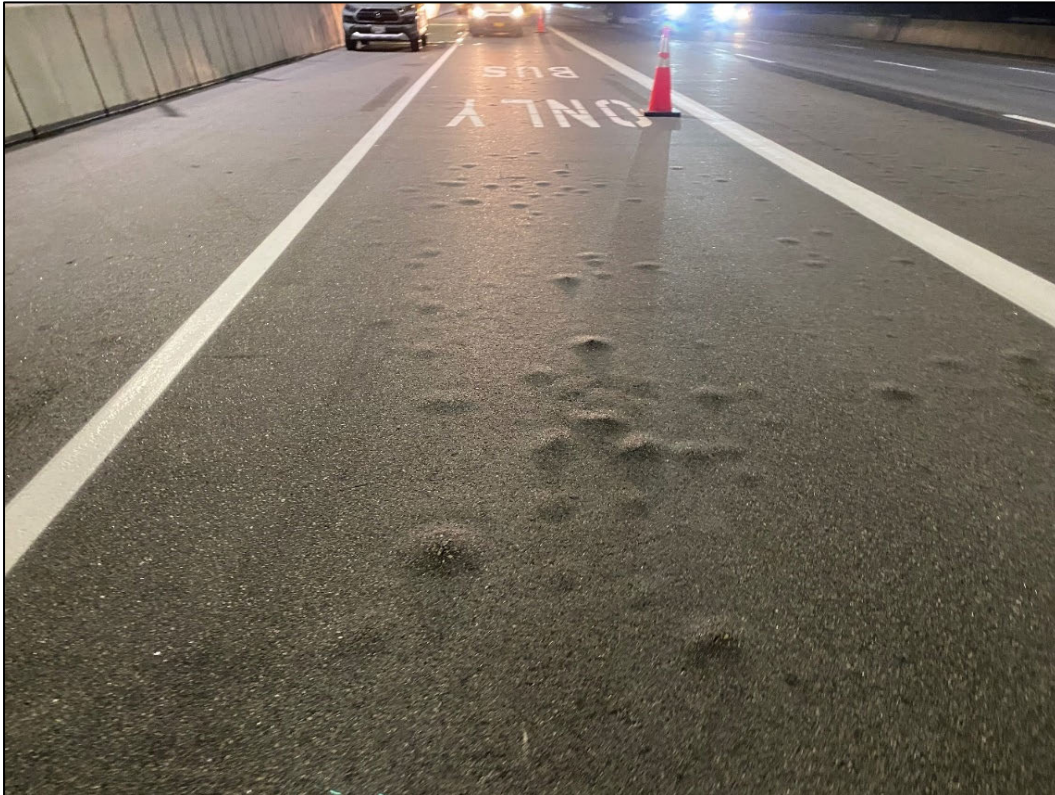
Figure 1. The “blisters” in question. Blisters are typically 4 to 8 inches and diameter and are observed throughout the bridge; however, the frequency of blisters varies from span to span.
